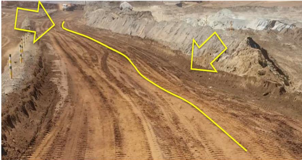
Figure 14 - Depressions on the runway
